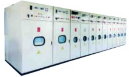
11KV Line Up Panels
